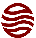
PHOTOGRAPH 22. Interior view of former Nettleton Planing Mill building. Old electrical panels on walls. Noted as former boiler room on historical Fire Insurance Maps.
