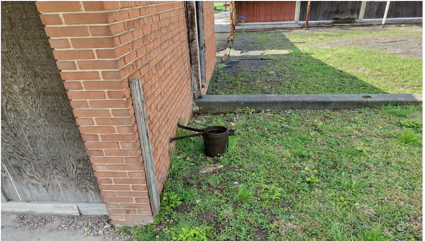
PHOTOGRAPH 15. Unknown underground piping located adjacent to former True Value garage building ( north face )
