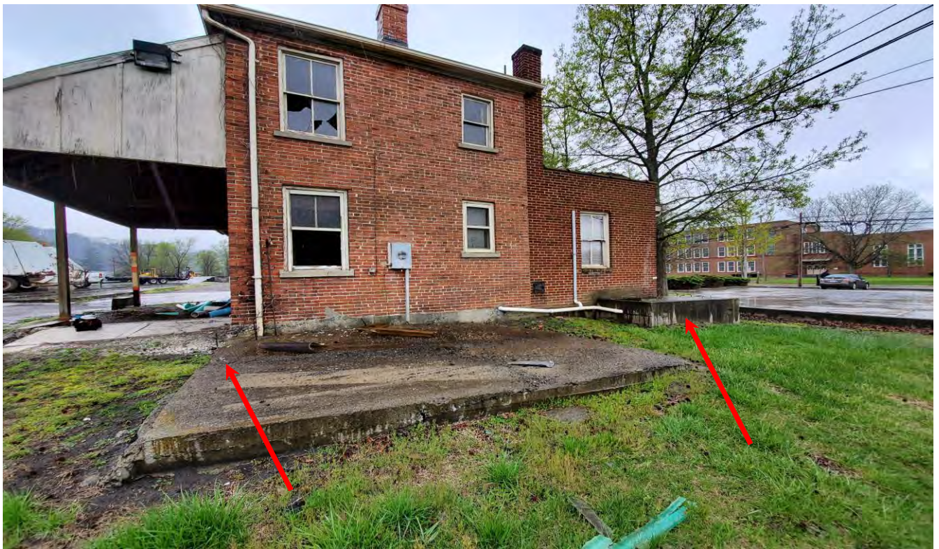
PHOTOGRAPH 3. Subject property. Former Nettleton office building ( north face ). Arrows point to legacy piping location and above ground septic tank.
