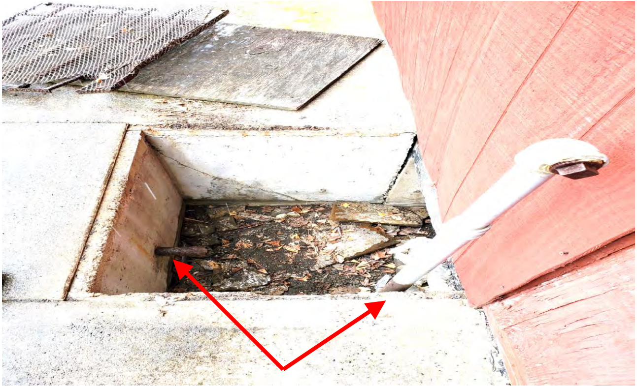
PHOTOGRAPH 11. Subject property. Legacy piping leading to basement boiler room.
