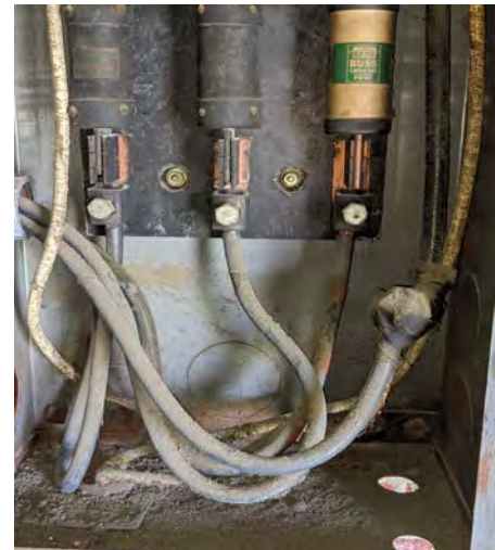
Assumed ACM wiring (Building 1 storage room)
