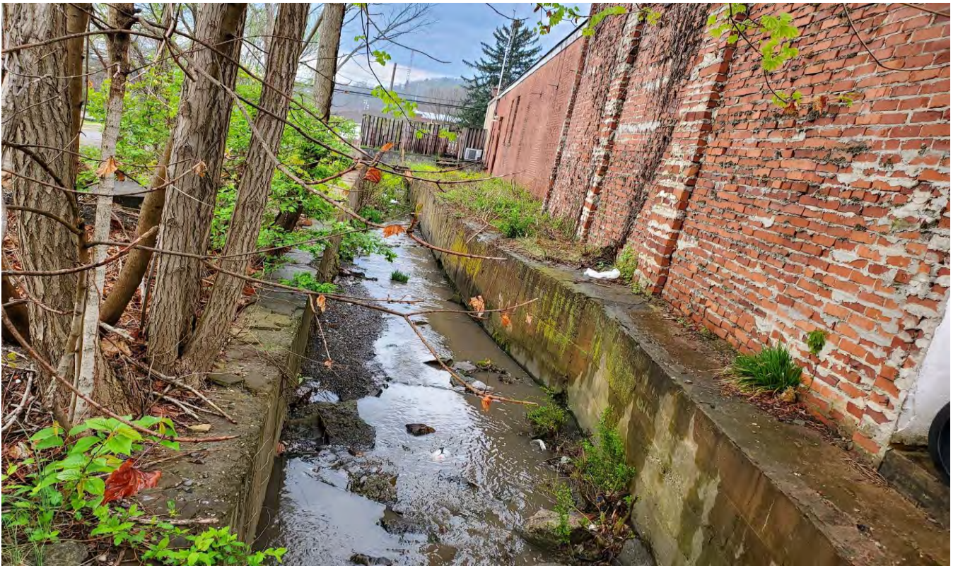
PHOTOGRAPH 8. Channelized drainage separating the subject property from adjacent northern property. Subject property left of photo. Water flows east to west.
