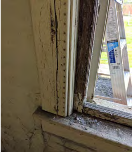
Sample 2-P-02 (LBP – Off white Window Casing)
