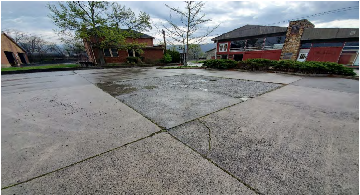
PHOTOGRAPH 10. Subject property. Parking area north of former True Value store building. Large square area of concrete center of photo appears to have been repaired.
