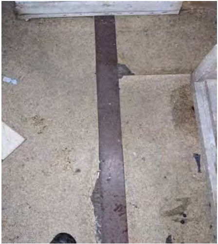
Samples 3-10 to 3-12 (Beige Flooring) and 3-13 to 3-15 (Brown Flooring Strip in center) - ACMs
